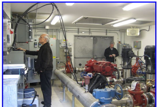
Booster & Fire Pump Station
