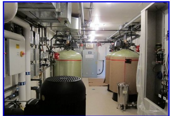
Mobile Water Treatment Unit
